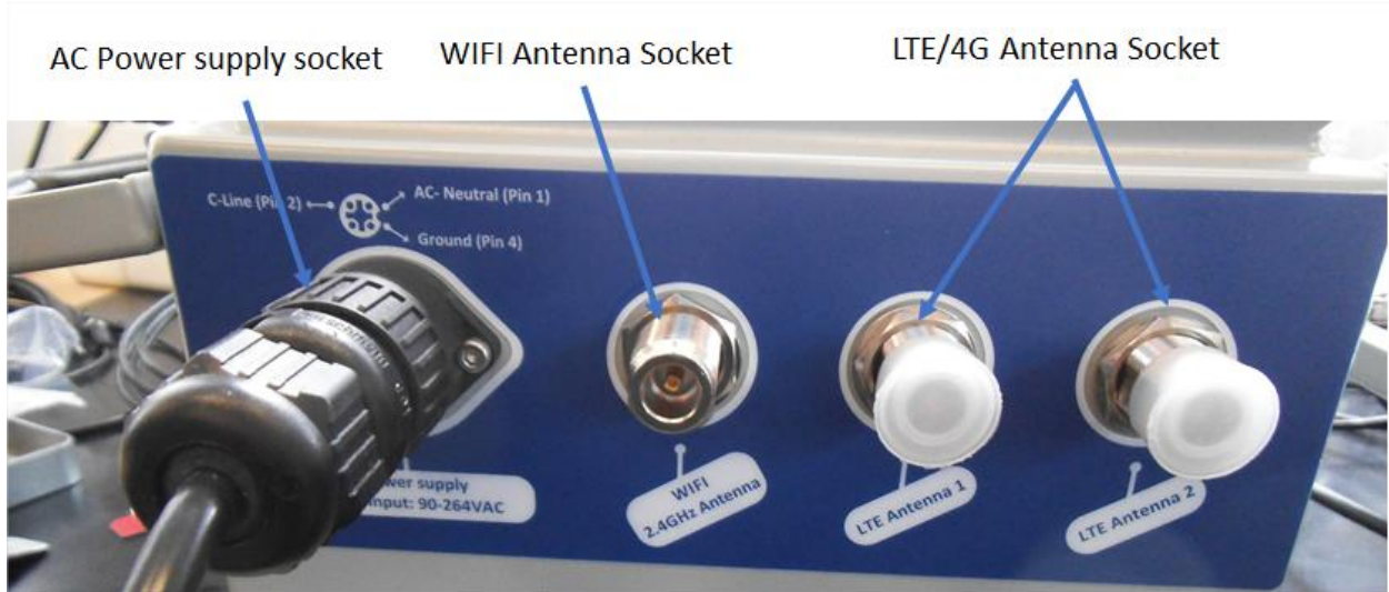
Figure 3 : Antenna and power supply connectors
