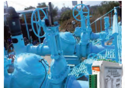
Water and Sanitation Wireless acquisition of basic variables measurement from the injection of current rectifiers for the cathodic protection of pipelines.
