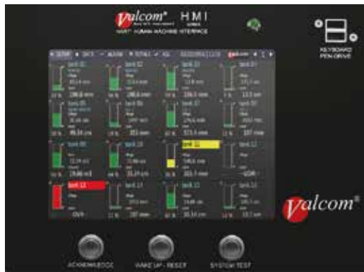
HMI Data acquisition and control panel
